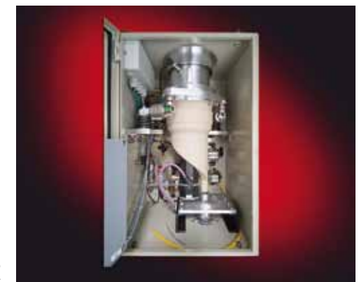
Internal view of the dosing equipment
