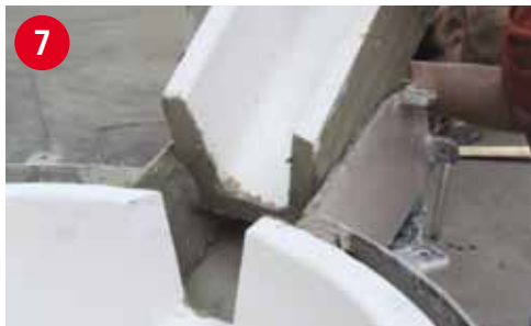
Steel shell around the spout is covered with INSURAL 800 mastic
