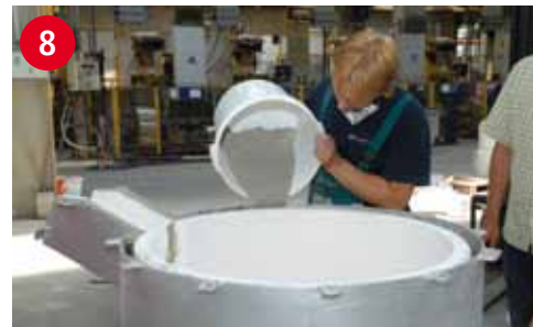
The gap is filled with the rest of the backing material up to the top, it is compacted and sealed with a layer of INSURAL 800 mastic of approx. 15 mm
